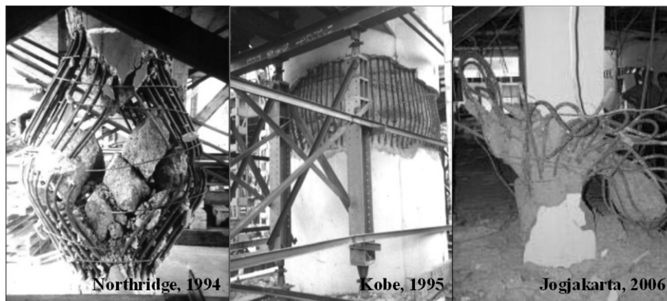
Fig. 1 The failure of structure in vertical earthquake
